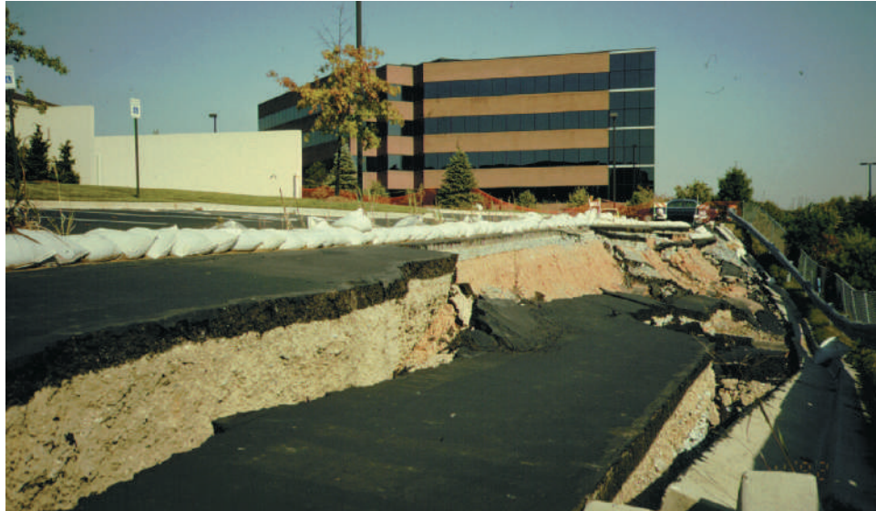
Figure 1.11 Better knowledge of the soils on which this road was built may have allowed its engineers to develop a more stable design, thus avoiding this costly and dangerous situation. (Photo courtesy of Ray R. Weil)
